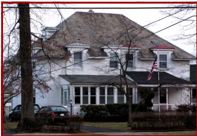
Original slate roofing maintained on two homes in the Harriman section. Twin homes on Wilson Avenue were formerly the Recreation Center for the Emergency Fleet Corporation, c.1918.
