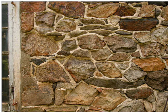
Illustration for Masonry Repointing: Detail of eighteenth century pointing. The most common joint profile type for rubble stone masonry was the raised ridge joint.
