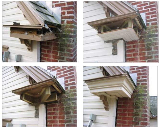
Illustration for Deteriorated and Missing Components. Sequence of restoration of a severely deteriorated cornice return. The crown molding was custom-cut for the project, a procedure that requires scheduling but does not add significantly to the repair cost.
