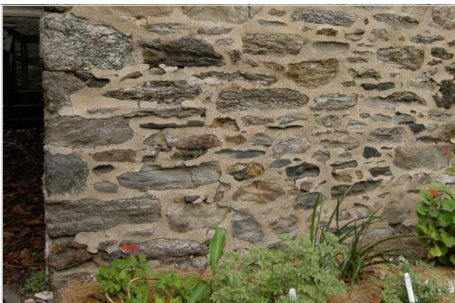
Illustration for Masonry Repointing: Overly-hard Portland cement mortar restrains the expansion of permeable stone masonry and results in the delamination (loss) of the face of the stone.
